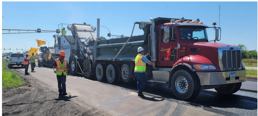
Truck lane paving at the southeast end of MnROAD's I-94 Interstate bypass mainline.
