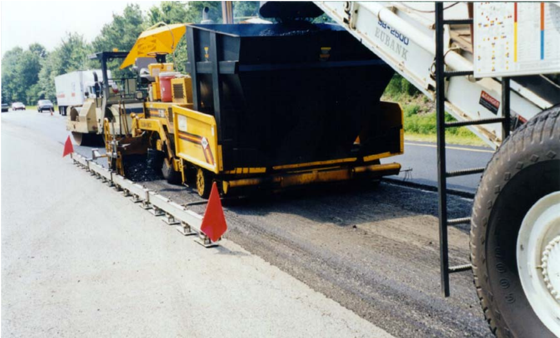
Figure 3. Pavement With No Tack Coat Prior to Placement of Mixture
