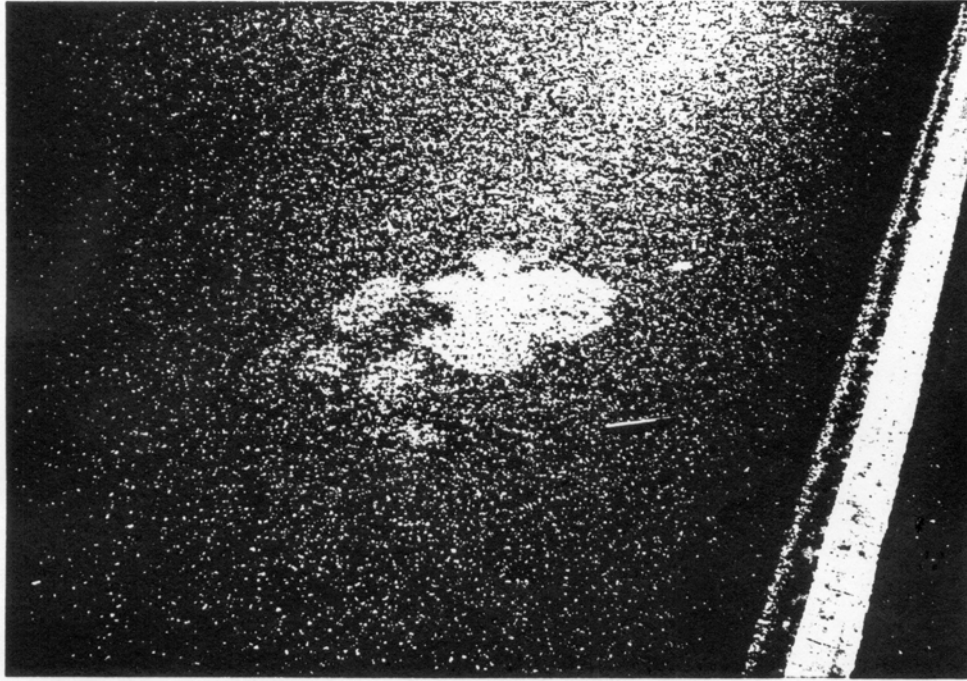
Figure 3. Typical Localized Bleeding Area, North Bound Lanes, I-55, Near Collinsville, IL
