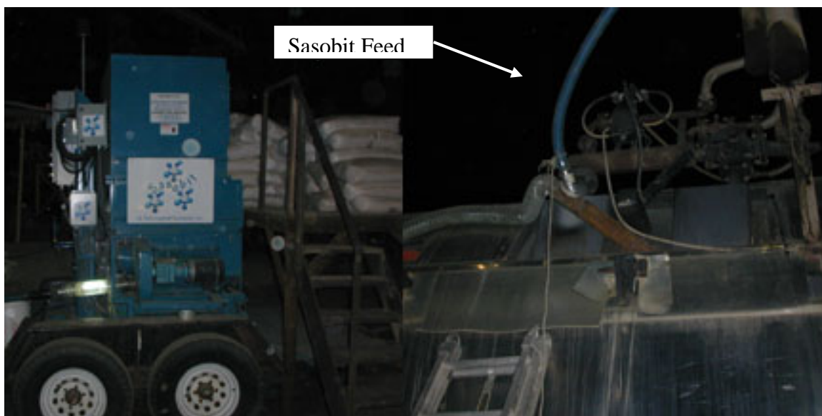
Figure 2. Sasobit® Pneumatic Feed to Mixing Chamber.
