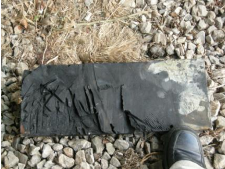
Figure 2.33: Bearing pad after forceful removal
