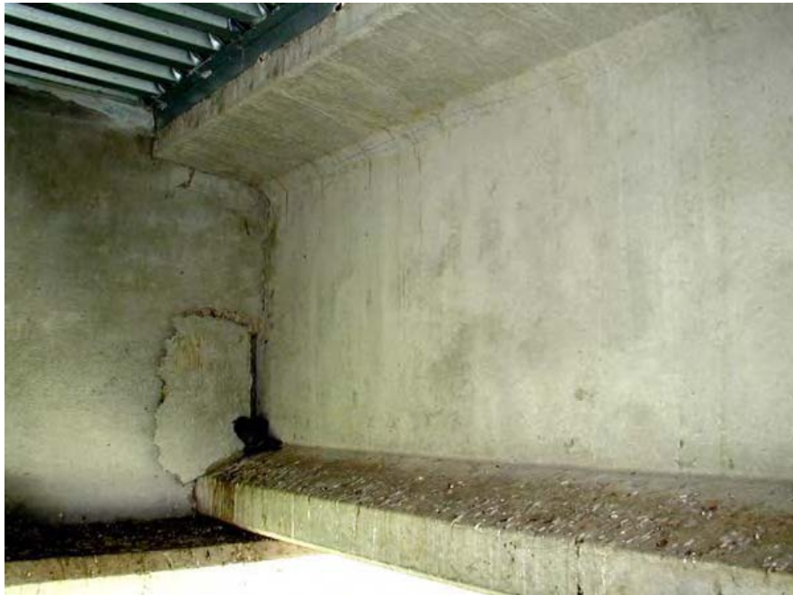
Figure 2.18: Typical diaphragm face crack (Swenson 2003)
