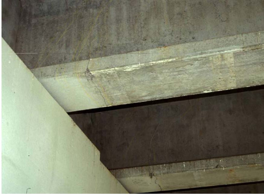
Figure 2.17: Cracked pre-tensioned bulb-tee girders (Barnes et al. 2006)
