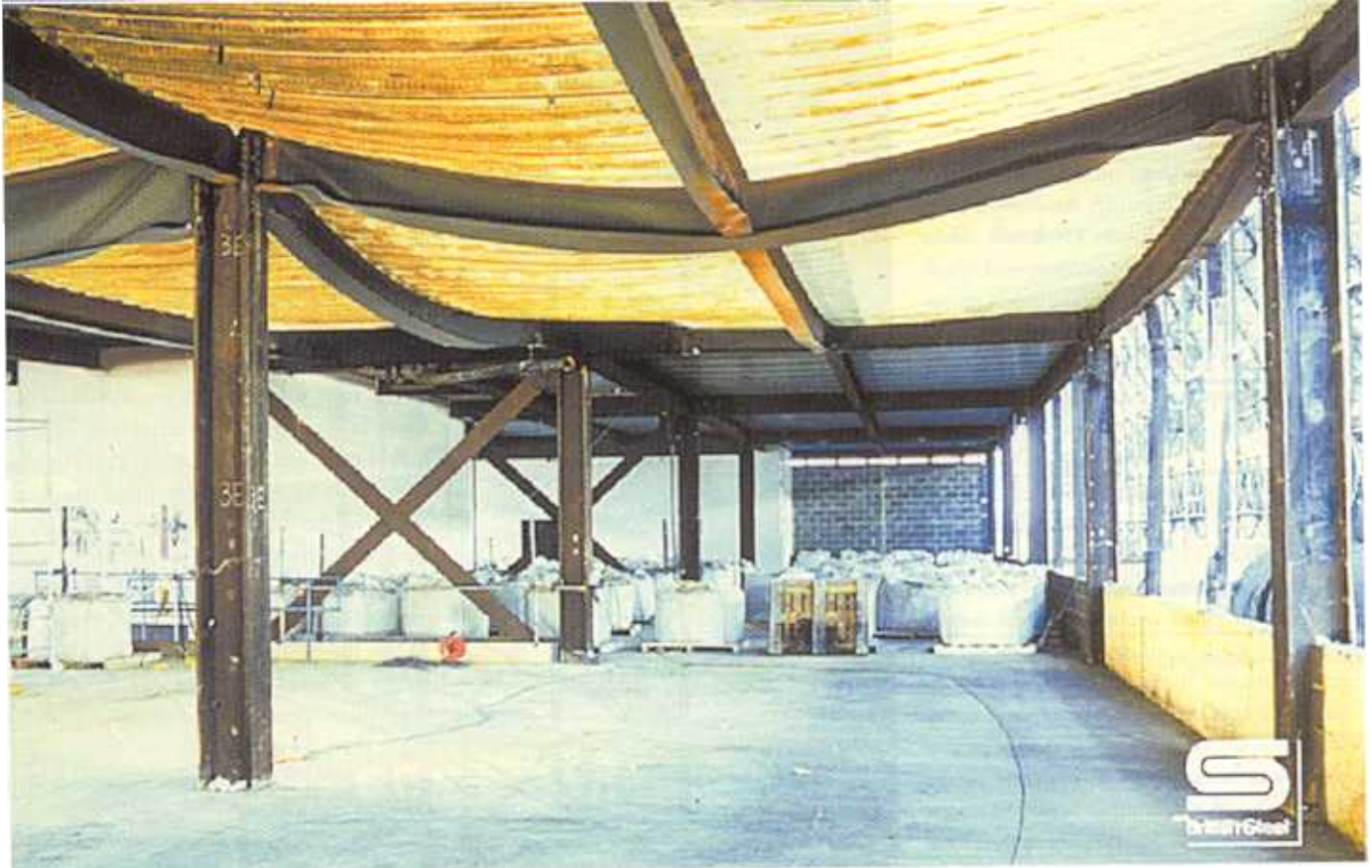
Beam in Cardington Tests after reaching temperature in excess of 1600°F.
