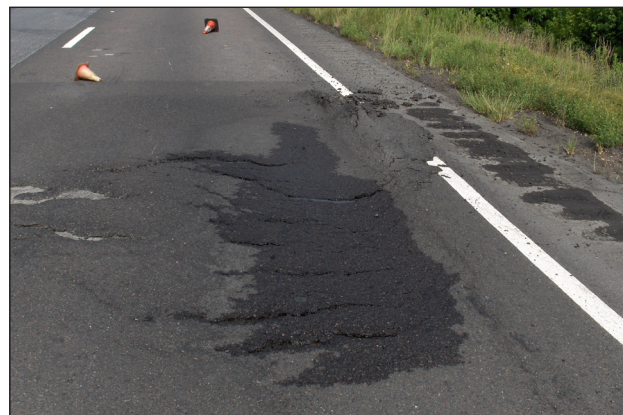
Figure 1 Severe pavement distress on Section N8 at the NCAT Pavement Test Track.
