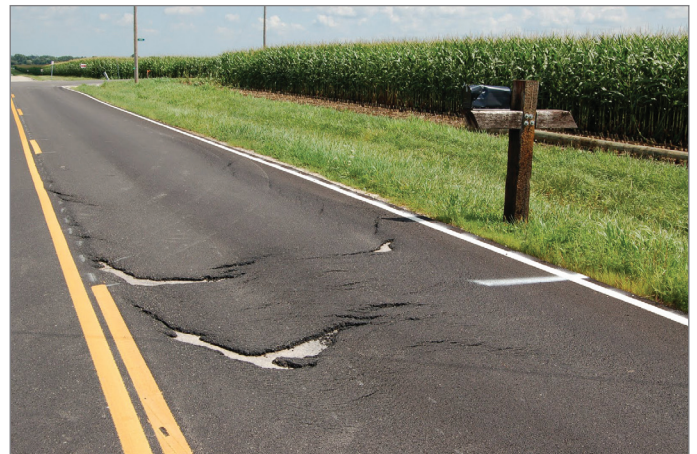
Figure 1. Example of pavement distress caused by debonding.
